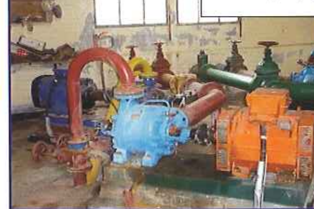
Station de pompage
